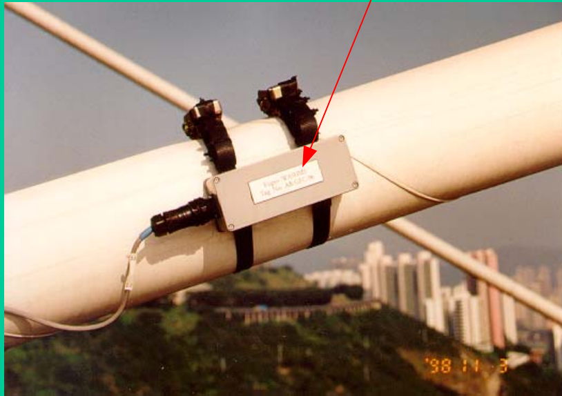
Accelerometers Mounted on Longitudinal Stabilizing Cable
