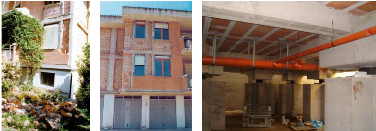
Fig. 19. Damage of the 1997-98 Marche and Umbria earthquake to the Fabiano house and new underground floor after the insertion of 56 HDRBs and cut of most old foundation piles (April 2005).
