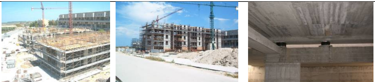
Fig. 20. Seismically isolated buildings under construction at Cerignola (in June 2005 on the left and in September 2005 at the center) and view of two of the 124 HDRBs installed at the top of their first floor.
