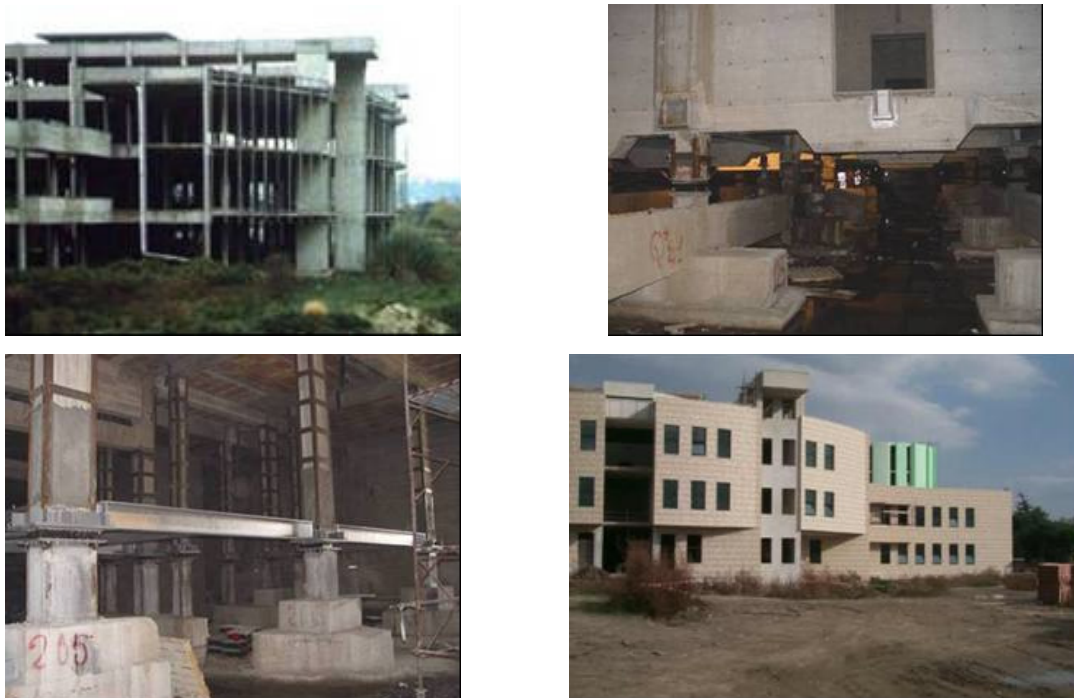
Fig. 18. Views of the Rione Traiano Civic Center at Naples after the structure completion in the years 1970s, of its foundation columns and walls cut during upgrading with approximately 630 HDRBs, of the new steel reinforcing floor installed above the isolators and of the upgraded building in 2004 (first retrofit with SI in the European Union – EU).
