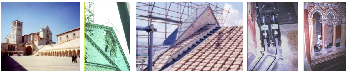
Fig. 21. The Upper Basilica of St. Francis at Assisi – From left to right: after its restoration; tympanum damaged by the first shock of the 1997 earthquake; during and after the installation of 47 SMADs between both tympana and the transept; during installation of the 34 STs.
